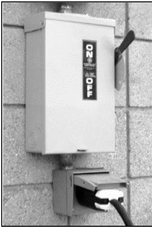
Figure 3. 240V electric outlets with NEMA 14-50 receptacles
